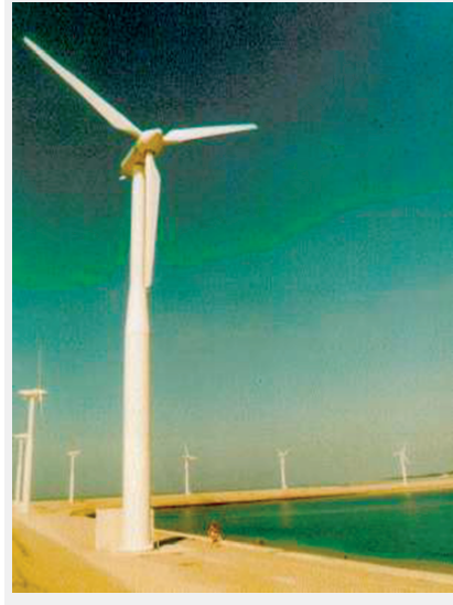
Fig. 8.70. To maximize the efficiency of a wind energy converter, the pitch controller must consider many inputs
