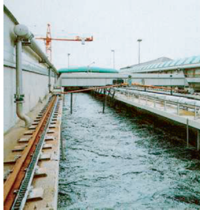
Fig. 8.63. By injecting \text{FeCl}_3 into the sludge, dissolved phosphate precipitates from the waste water
